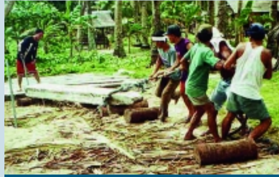
Concrete slabs for the seawall were moulded and hauled manually by the volunteer working groups.
