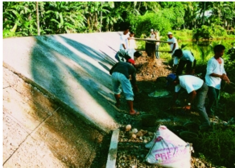
The CBDP process often leads to construction of physical mitigation measures, and the LGU should, preferably, contribute technical expertise and materials, while the community invests volunteer labour.
