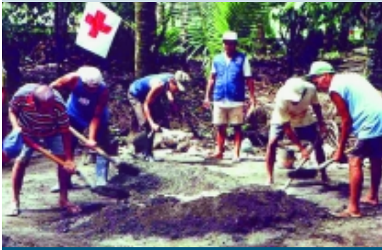
Community volunteers work in shifts, so each group only needs to allocate one day per week to the construction work.
