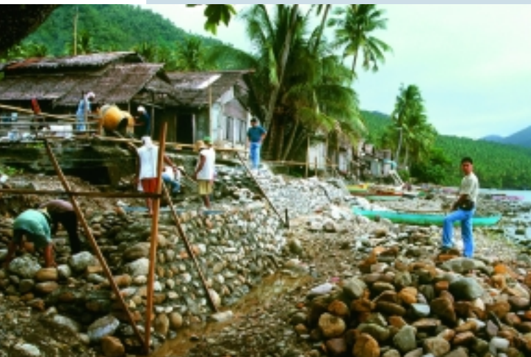
The volunteers work on building the protection wall along the beach front.
