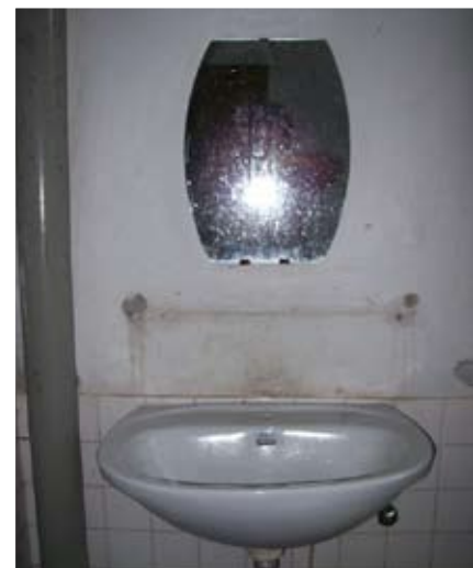
This sink is in a new District hospital. It is the only washing facility for out-patients and yet it has not been plumbed in.
