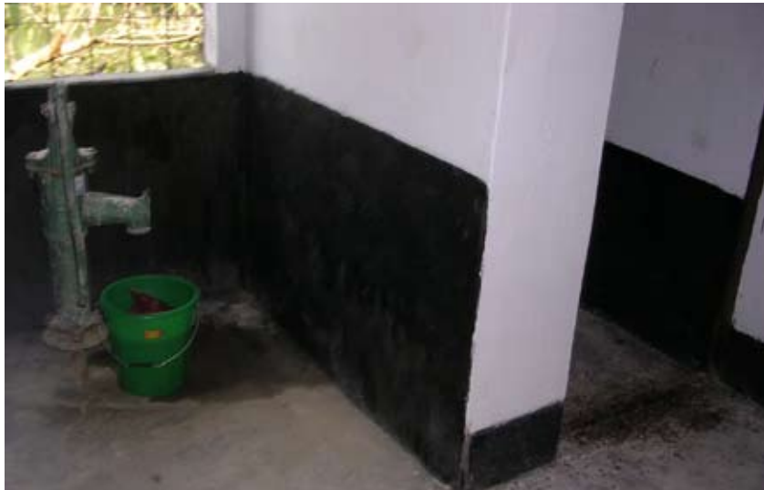
The tube-well at the newly opened Community Clinic is not working (Rural South)
