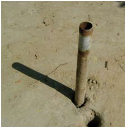
A deep tubewell has been sunk on the grounds of the Government Primary School, but it is faulty and has been abandoned by the construction company.
