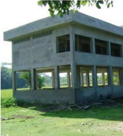
Soon to be extension of Government Primary School, a new construction under PEDP II.
